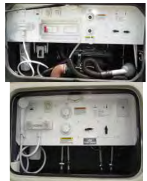
Fig. B - Utility Center
