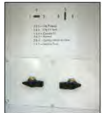
Fig. A - Water Valve Controls
