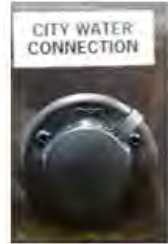
City Water Fill with City Water Connection Label
