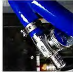
Fresh water drain valve
