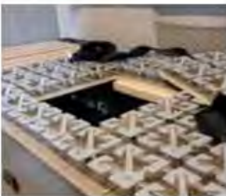
Water heater Bypass Access
